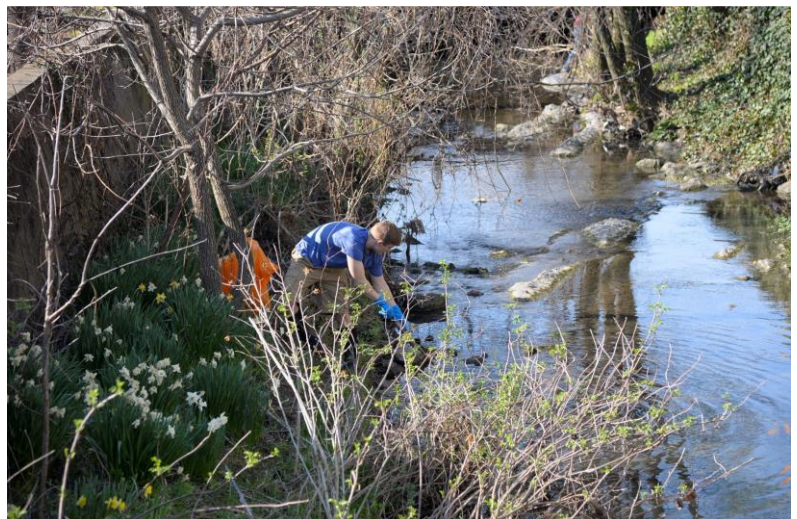
(Above) An unidentified man performing stream restoration efforts at a stream in Harrisonburg.
