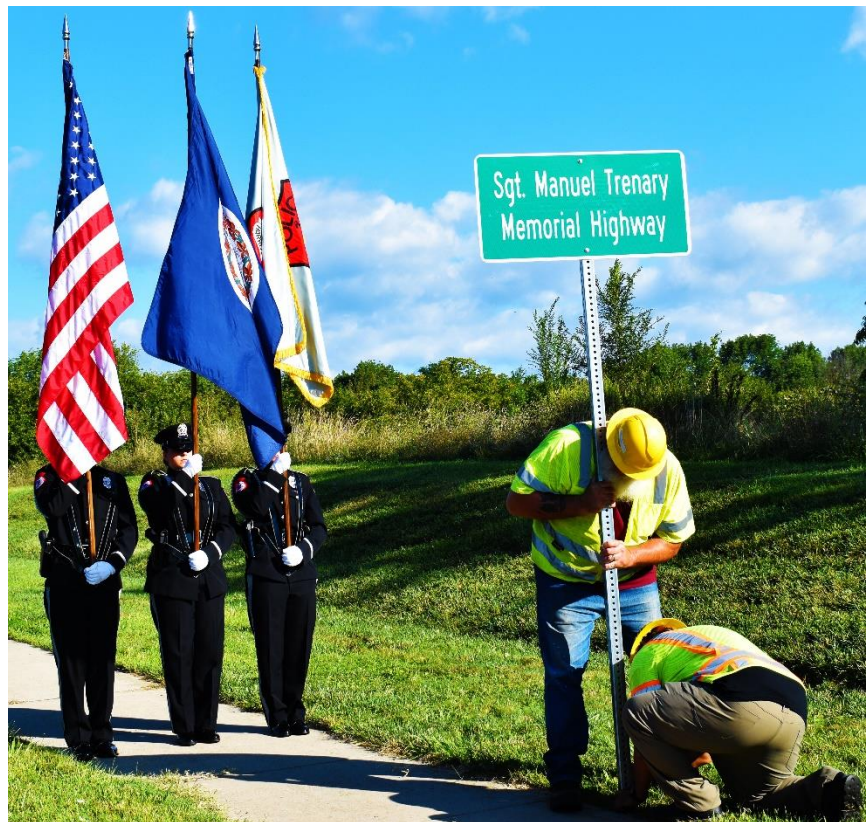
(Above) Members of the HPD Honor Guard watch as Harrisonburg Public Work staff install the new sign honoring Sgt. Manuel Trenary on Erickson Avenue.
