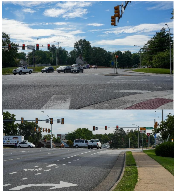
Crews will begin demolition and construction of the sidewalk ramps at the intersection of Port Republic Road and Main Street (top) starting Tuesday, Aug. 9. The northbound Main Street slip road (bottom) will be closed to thru traffic for the duration of the construction project.
