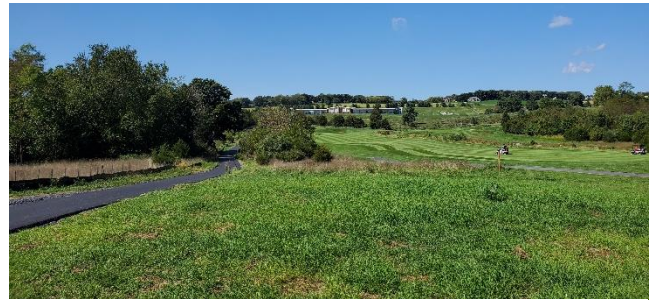
(Above) Construction on the path started this spring. It likely will be complete later this year.
