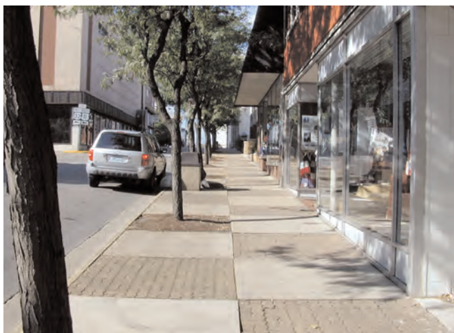
The present, 1970’s era streetscape checkerboard paving pattern is hazardous due to differential settling and stylistically inappropriate for the historic downtown center.
