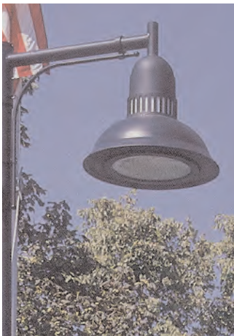
Retrofit fixture for cobra light.
