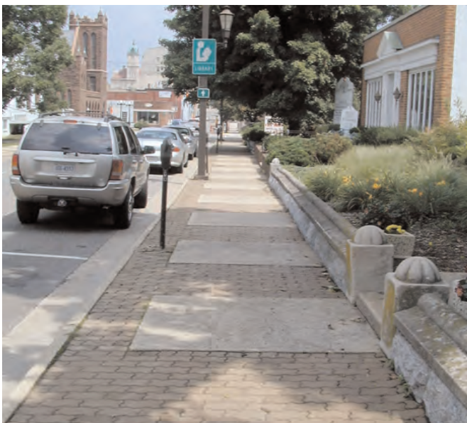
Section of South Main Street sidewalk converted in 70's to checkerboard unit paver/poured concrete pattern. Proposed Garden District sidewalks to be simplified to an all poured concrete standard.
