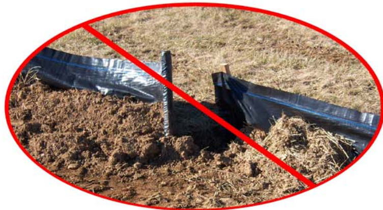
No gaps in silt fence.
