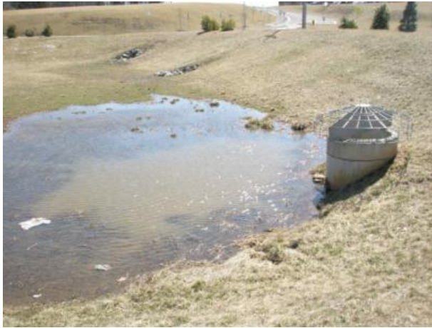
Figure 1: View of riser structure and standing water
