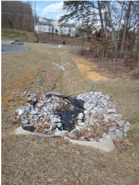
Figure 1: Erosion downstream of outfall
