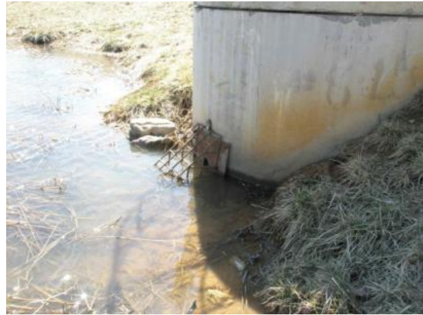
Figure 2: Close-up view of extended detention orifice and trash rack (water surface at the invert of the orifice)
