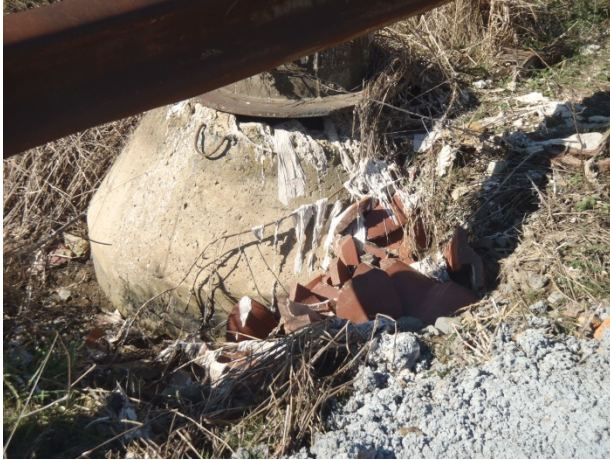
Figure 1: Leaking sanitary sewer line
