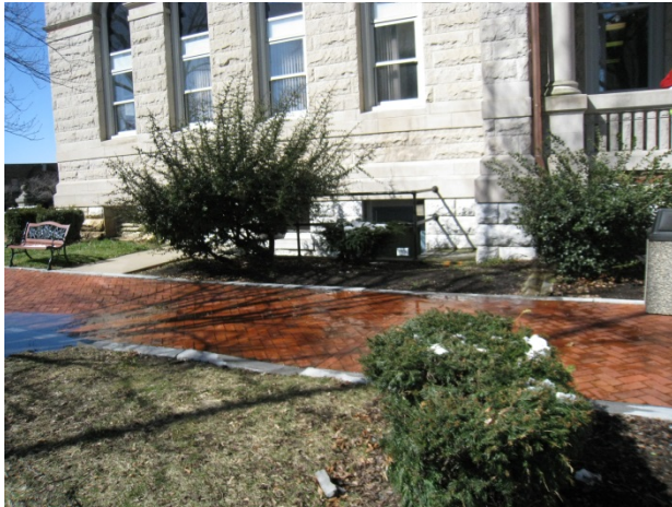
Figure 1: Planter bed & downspout in background
