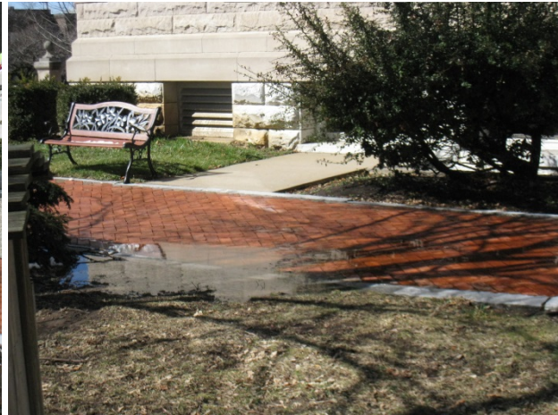
Figure 2: Water ponded on walkway and grass
