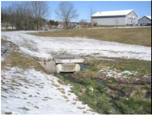
Figure 1: Principal Spillway. 2-year rectangular orifice showing (one each side); WQ orifice is buried 15" below rectangular orifice.
