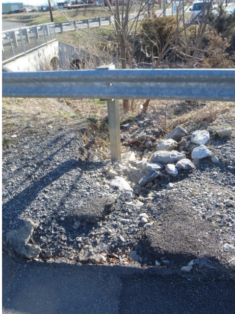
Figure 1: Stream bank erosion
