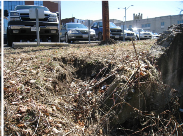
Figure 2: Close-up of erosion along bridge abutment
