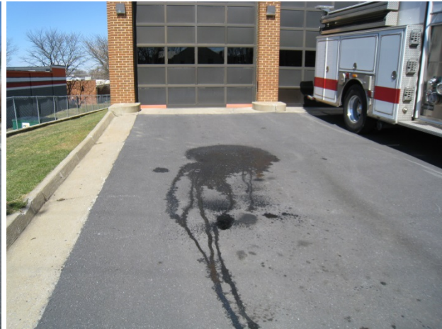
Figure 2: Fresh oil stain leaking to street
