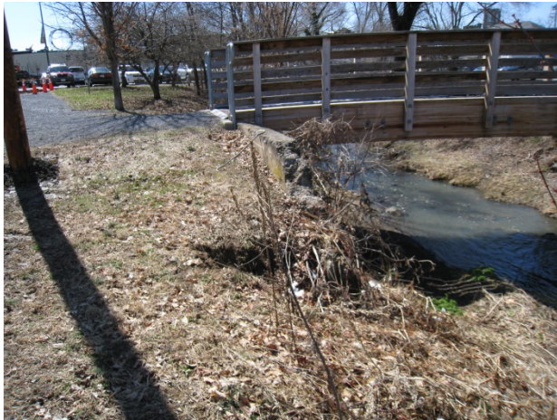
Figure 1: Erosion in front of foot bridge
