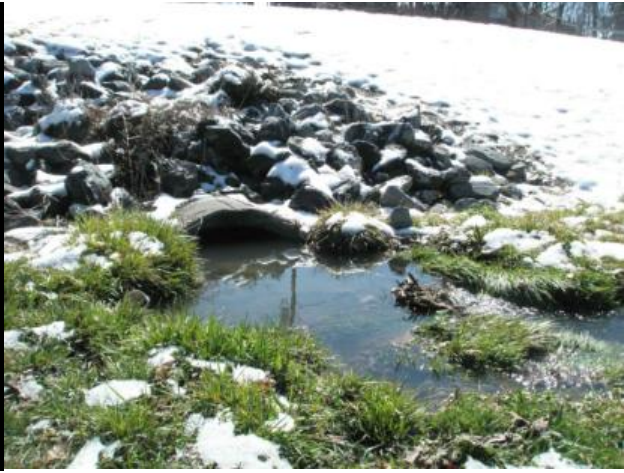
Figure 2: Inflow from diversion manhole in South Dogwood Street (basin silted in to top of pipe).
