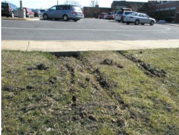
Figure 1: Parking lot contributing drainage area and existing erosion
